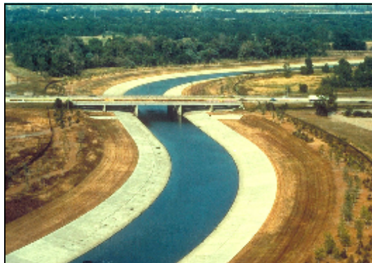
An example of river channelization: River Rouge in Dearborn, Michigan, USA. Photo from U.S. Army Corps of Engineers Digital Visual
